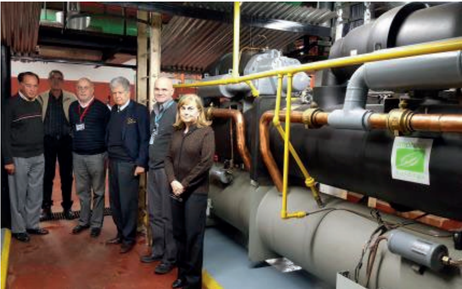
ARGENTINA: Non-ODS chillers provided to two hospital beneficiaries
